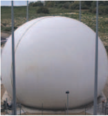
A gas holder: methane gas produced is re-used to provide heat for the treatment processes.
