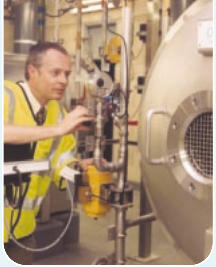
Water goes through extensive treatment processes before it reaches your taps
