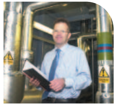
Our Combined Heat and Power Plant at Goddards Green
