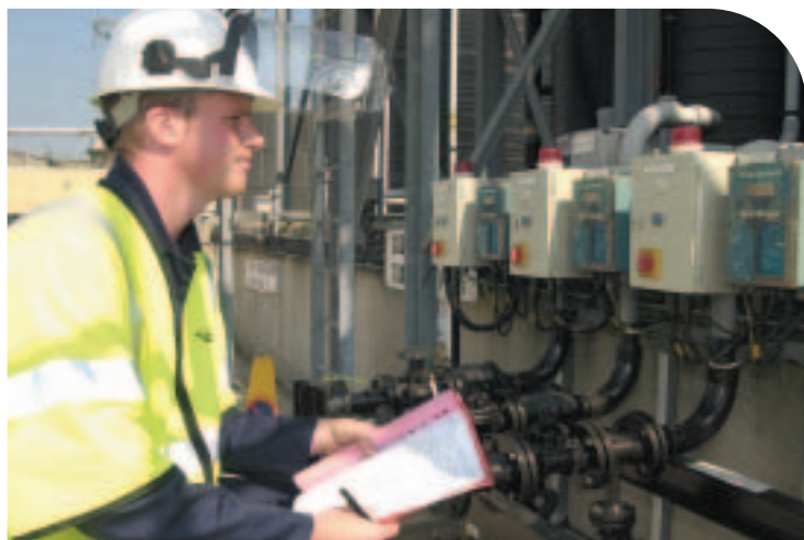
Monitoring chemical use at Millbrook Wastewater Treatment Works
