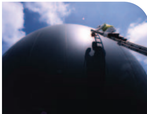
A methane gas holder at Worthing Wastewater Treatment Works
