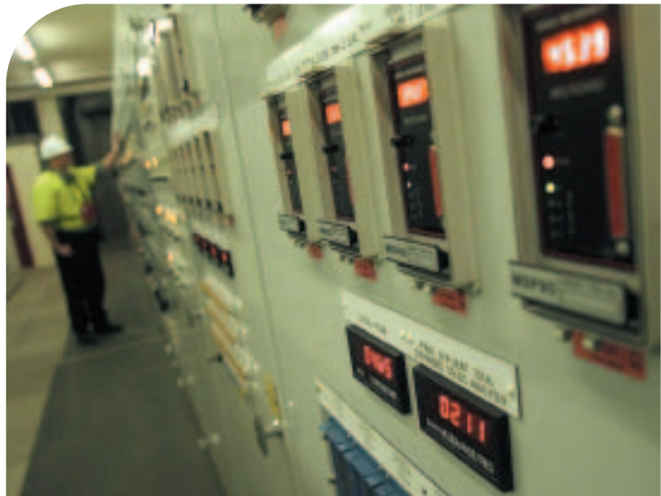
The control room at Eastbourne Wastewater Treatment Works
